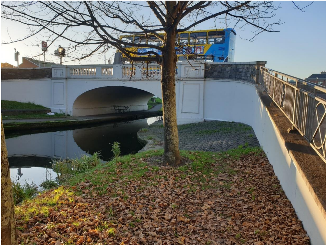
Existing Robert Emmet Bridge – looking from the East side. Location of proposed Kimmage 04 upper ramp
